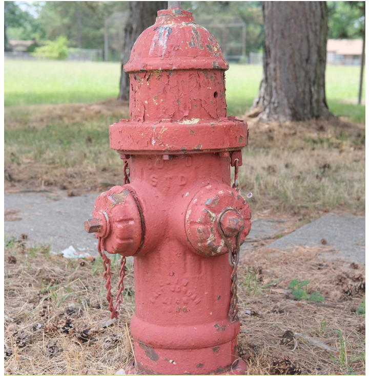
Hydrant , Charter Township of Royal Oak
