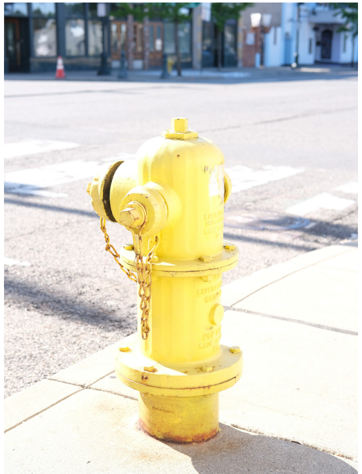
Hydrant, City of Pontiac
