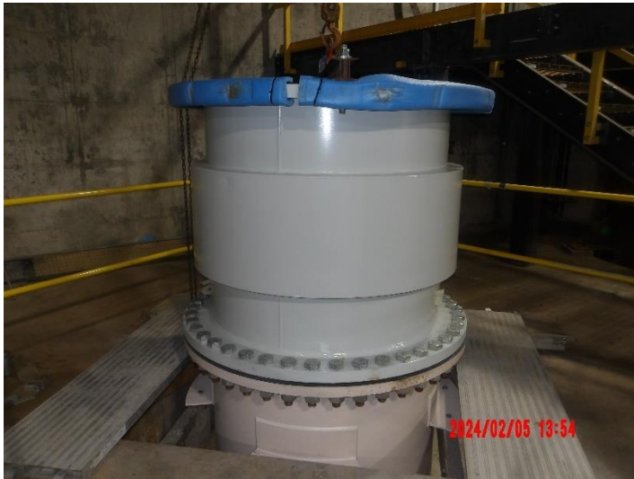
New magnetic flow meter at Pump #5
