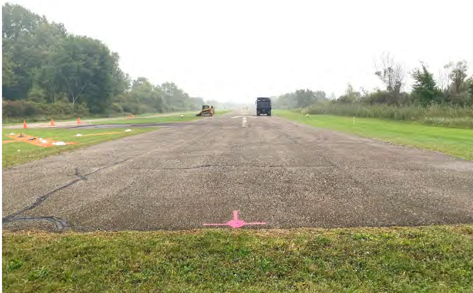
Photo 4. Conditions in Runway 8 APE, facing east
