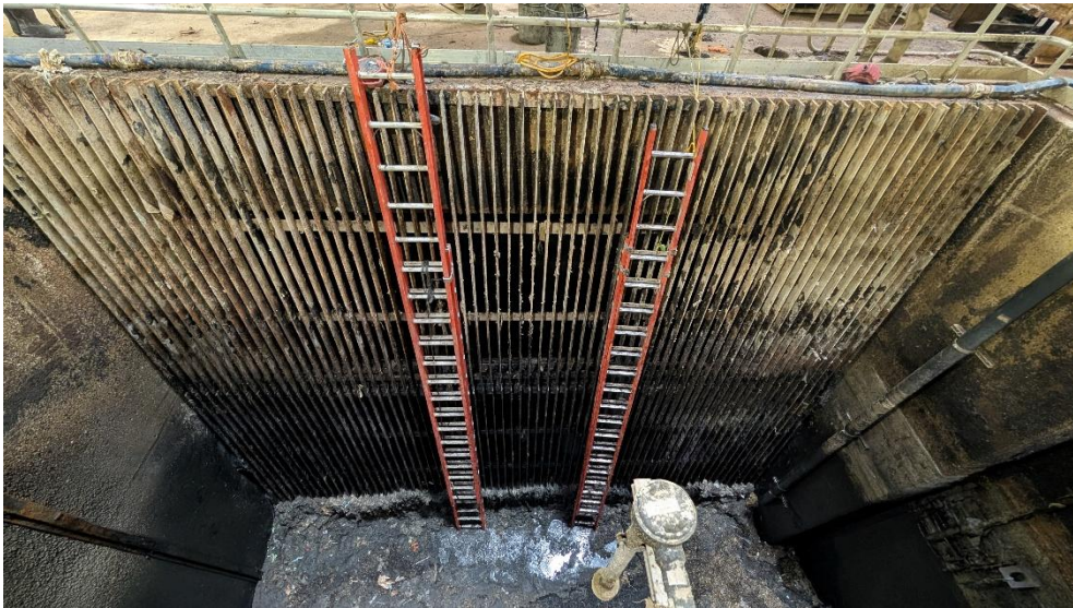
South side wetwell bar-screens after cleaning
